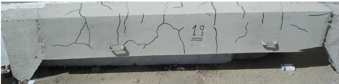
Figure (11) Crack pattern at failure for column C2.
